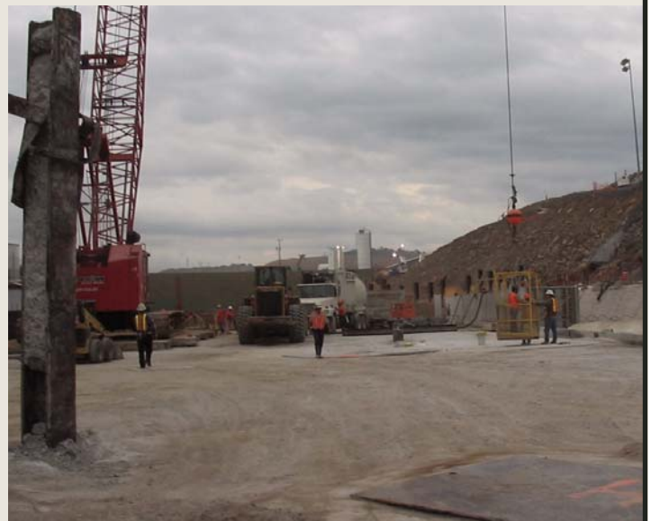
Once the work was completed and all the concrete was removed, covers were placed over the holes that remained.
