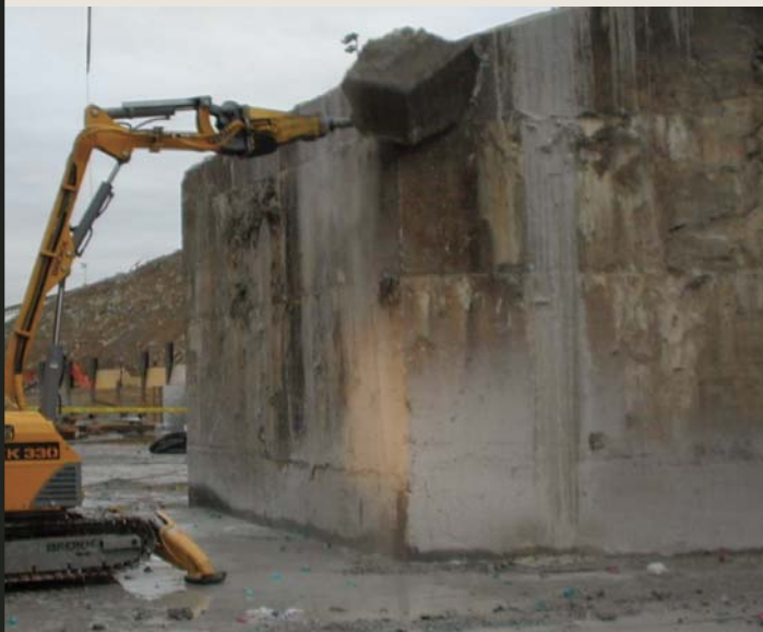
Once the cutting stage was completed, a Brokk robotic hammer was used to break up the concrete.
