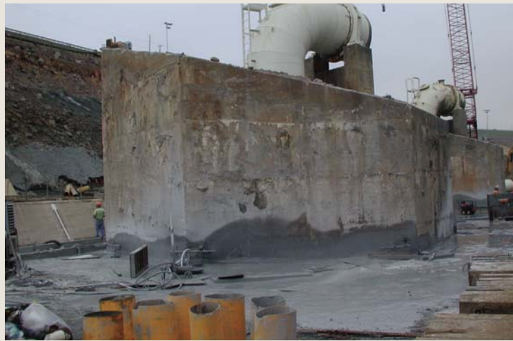
Each 40-foot riser pier was cut by a diamond wire saw before demolition could be completed.
