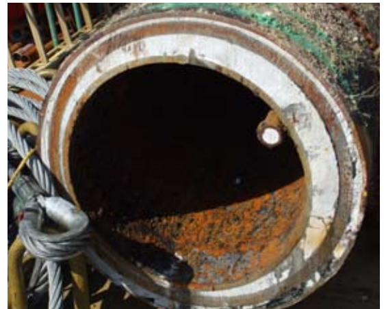
A 33" conductor segmented at a 125' depth offshore in the Gulf of Mexico.
