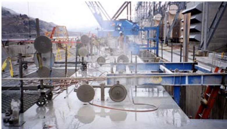
Multiple diamond wire saws performing precise cutting techniques for fish bypass system at Rocky Reach Dam in Wenatchee, Washington.
