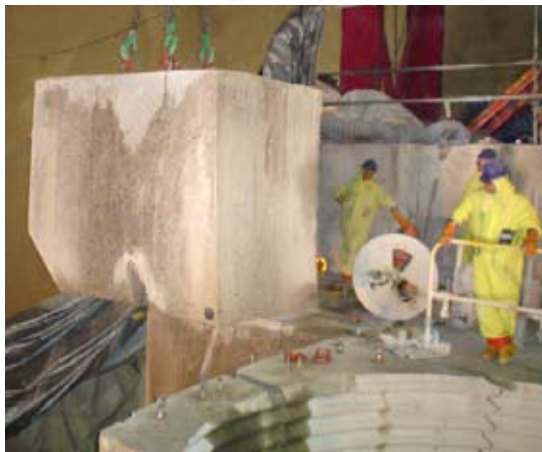
Removal of a 20 ton concrete block at Big Rock Point in Charlevoix, Michigan.
