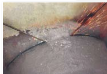
Nozzle cut at completion. Average cutting time for the six nozzles was 22 hours. No water or other liquid coolants were used. This minimized waste, and simplified the cleanup process.
