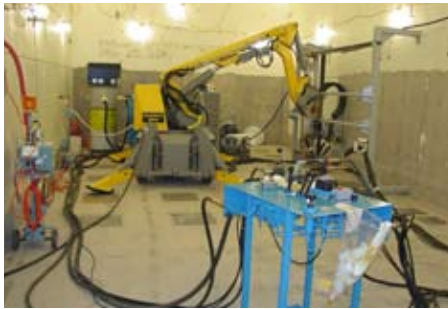
The Bluegrass wall shaver (shown above) and floor shaver (shown above right) was used in the Rocky Flats decontamination project.
