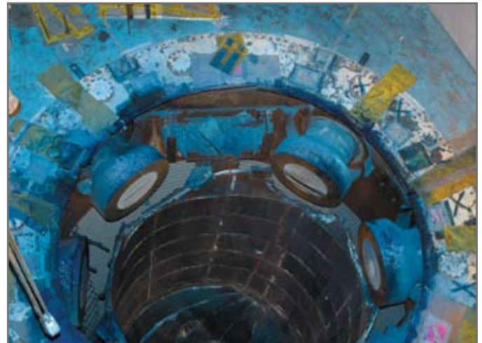
Fig. 11. Nozzle cut after completion. The nozzle measured 53" in diameter and had a 12" thick carbon wall with 1/2" thick stainless cladding.
