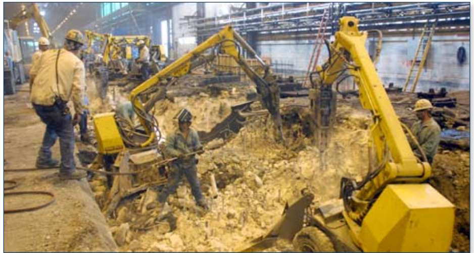
Demolition of the 600 cubic yards of concrete was completed in 4 days at NNII roll line.
