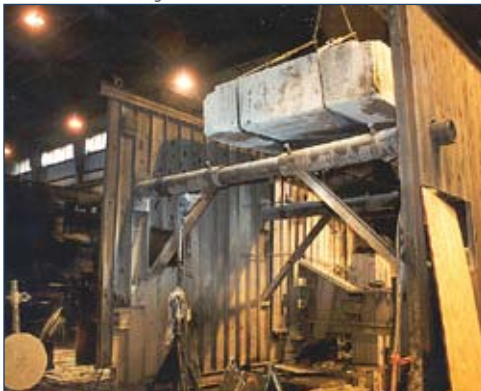
Fifteen ton concrete section wire sawed and removed from old foundation while the mill was in operation.
